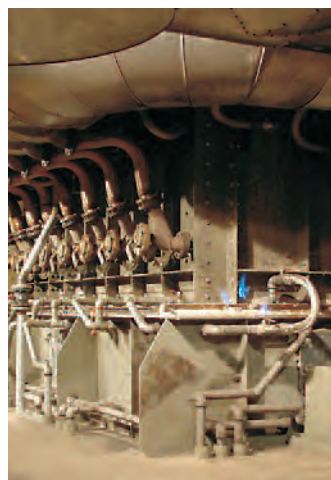
Black copper shaft furnace MKM, Hettstedt/Germany
